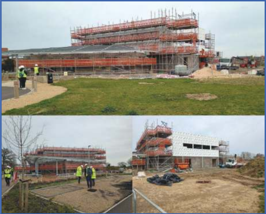
The Jubilee Centre from Walpole Crescent (top), from the nursery end (left) and from the southern football pitches (right) showing the main hall
