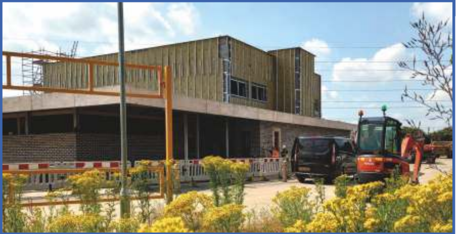
The Jubilee Centre in July. Top—from the south showing final cladding finish for sports hall, with nursery in front; bottom—from the north awaiting cladding. showing entrance area into reception and changing rooms below.
